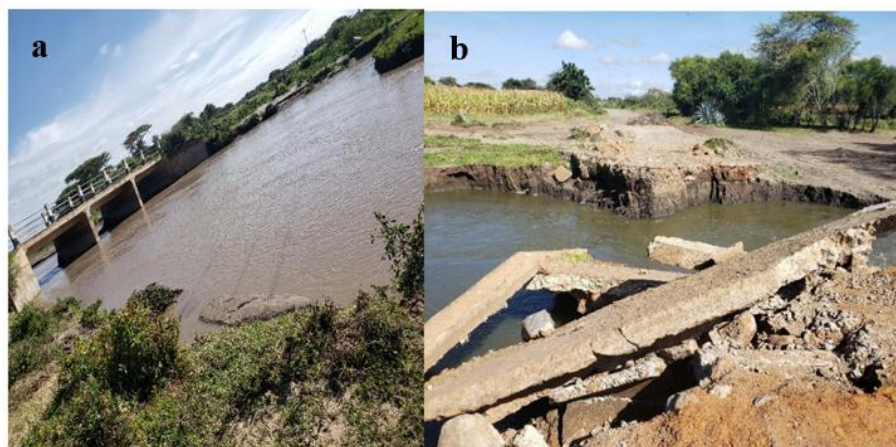
Figure 10: Turbid inlet water at Dongobeshi stream (left) and collapsed bridge at Gulidafia outlet stream showing sediment build-up and erosion impacts (right).
